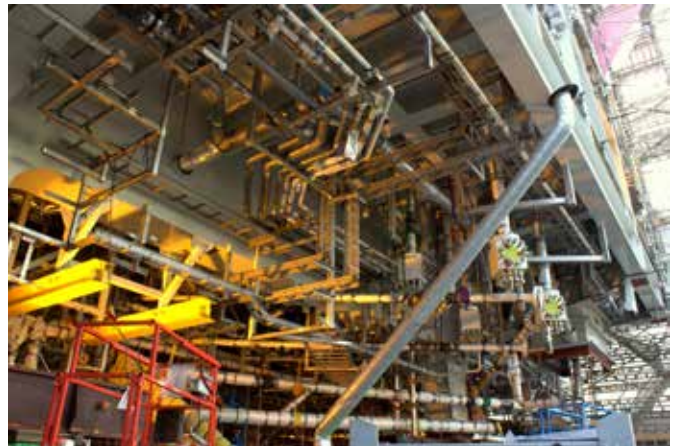
Above: Naturally, the area below a drilling module is very complex. In addition to the actual steel frameworks, there needs to be room for all the equipment, pipework, cable trays, etc. to fit in without getting in each other's way.
