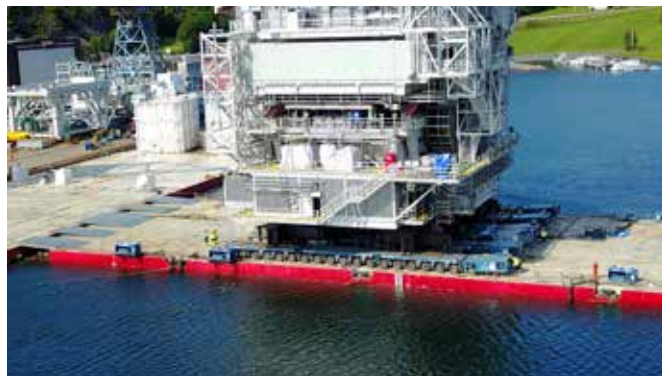
Above: The completed drilling module being driven out onto Boabarge 43 on Sarens SPMTs (108 axles)
