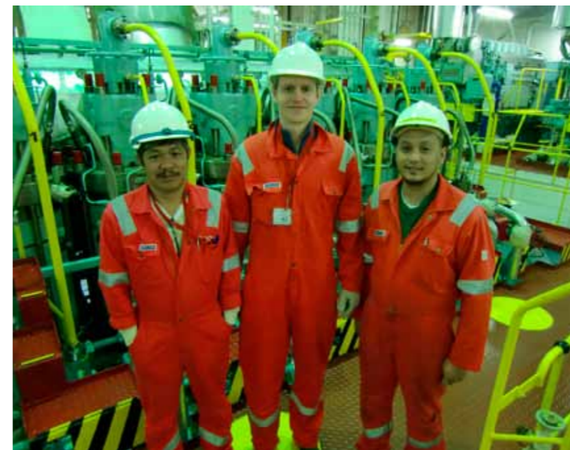
I maskinrommet/In the engine room. From left: Chief engineer William Noel, Øyvind Bjørnskau Johannesen and second engineer Remy Padilla.
